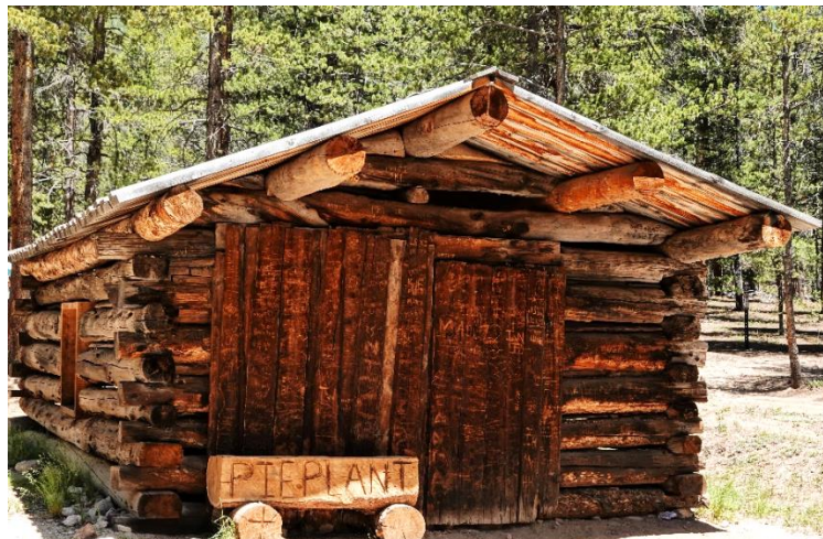
Figure 2. In 2006, the Forest Service and Passport in Time put a new roof on this Pieplant cabin in their preservation efforts. Photo date 7/2020 by S. Veatch.
