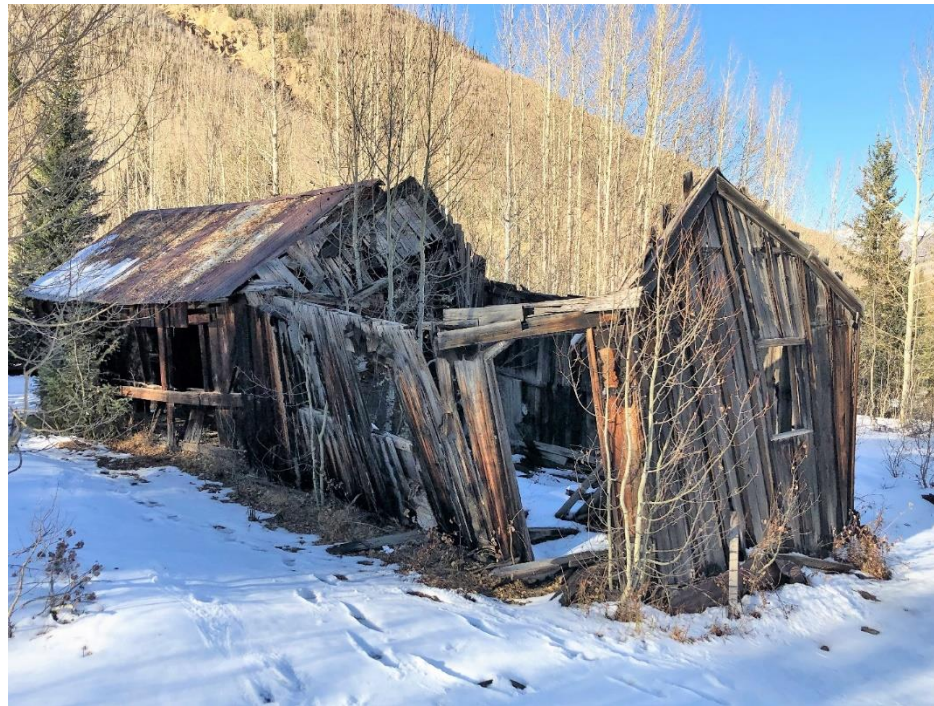
Figure 13 A miner's cabin and shed in Ironton. The roof of the shed has collapsed from the weight of many winter snows. Photo date 2020 by S. W. Veatch.
